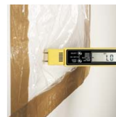
Plaster moisture contents
